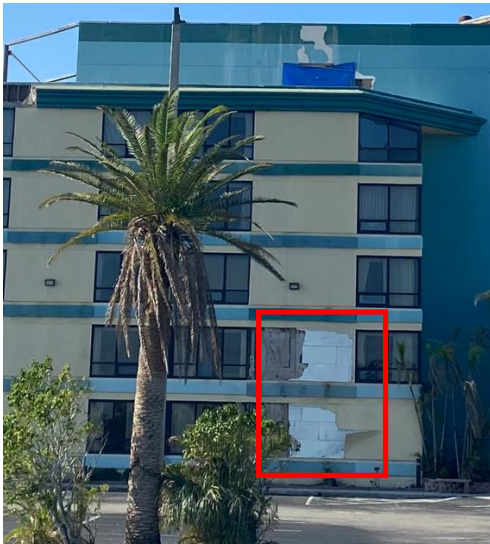
Figure 2: Cladding and opening protection damages
